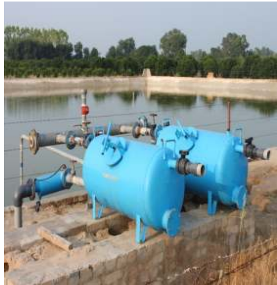
Micro Irrigation system Installed with Pond
