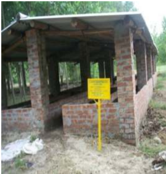
Vermi Compost unit at Abohar
